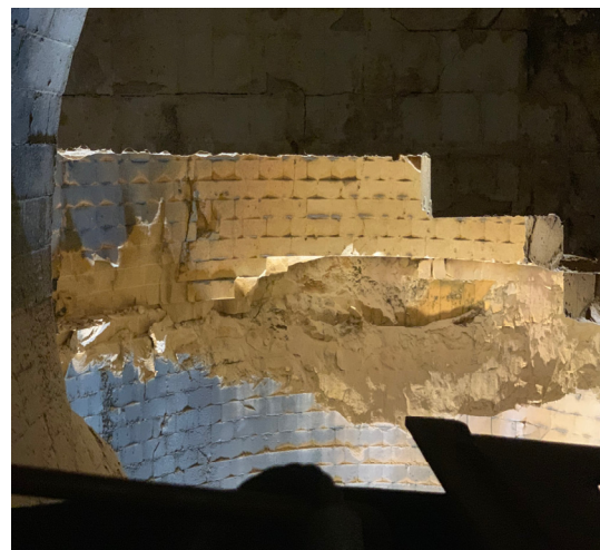
Fig.9. The status of the ceramic welding area after the cooling down of No.31 hot stove on July 5, 2019.
